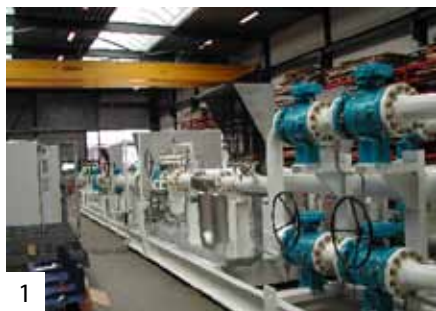
1 Process design and mechanical design of measuring stations for custody transfer of fuel, oil, diesel, natural gas and high purification chemicals such as hexane, butane and synthesis gases.
