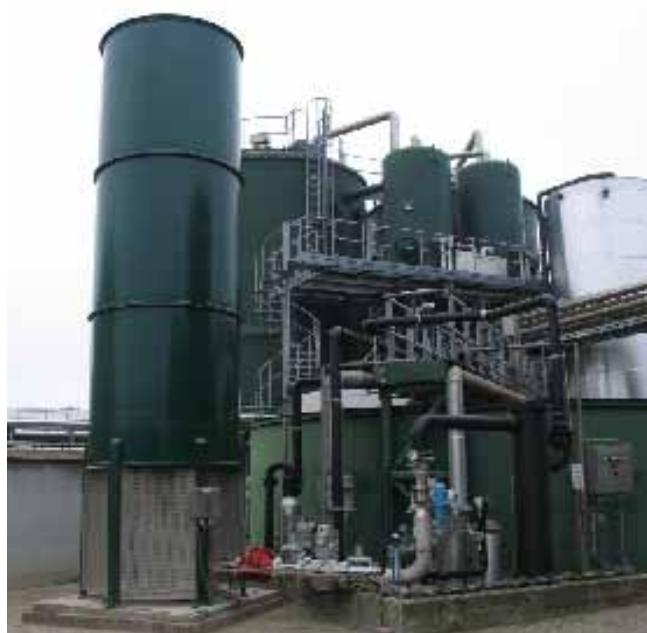
NER Flare Installations in operation
